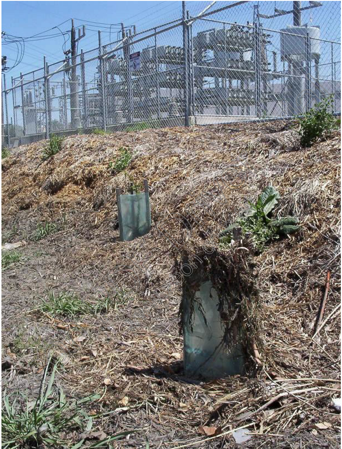
Debris on a tree-guard, about 1.5 to 2 metres below No3. Capacitor Bank
